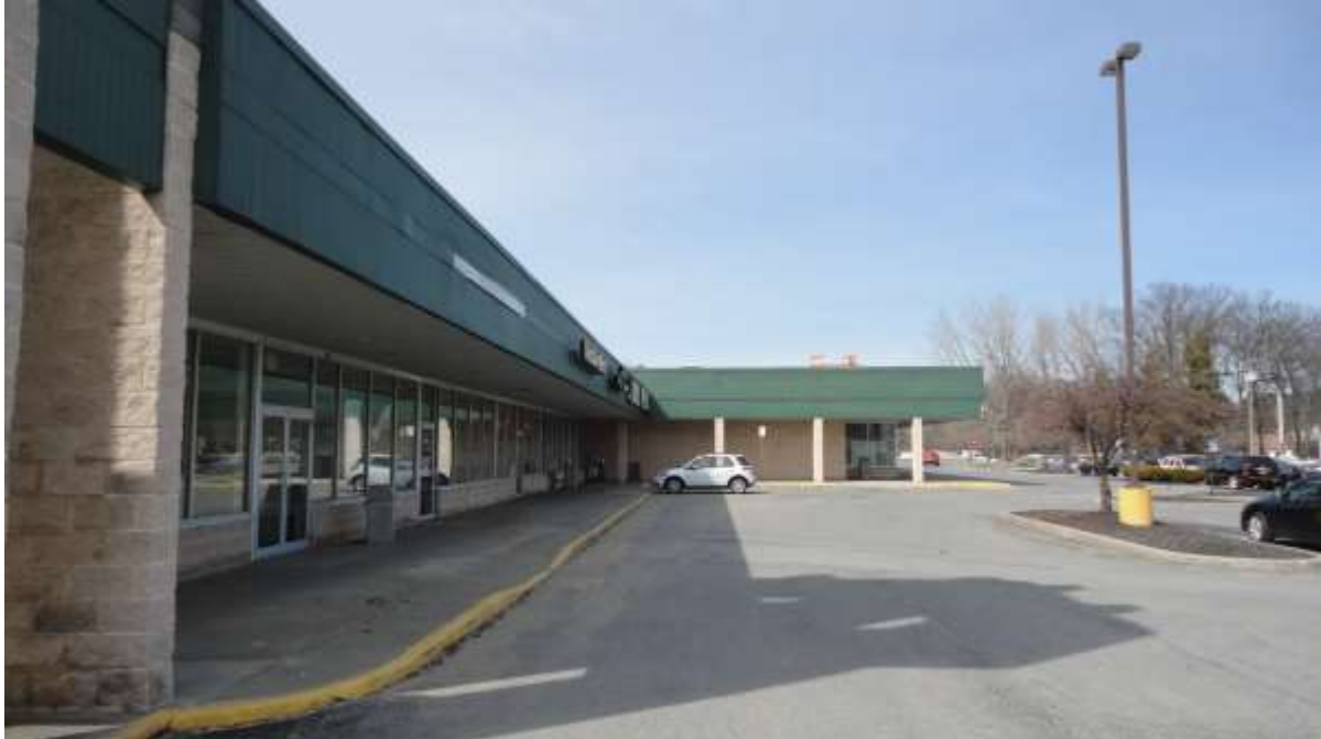
Existing sidewalk, storefront and cantilevered facade details on West Ave. south tower.
