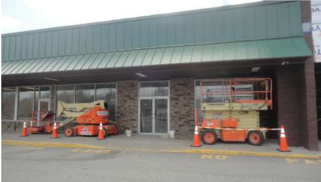
West Ave. façade with new metal siding and awning, and new stone veneer.
